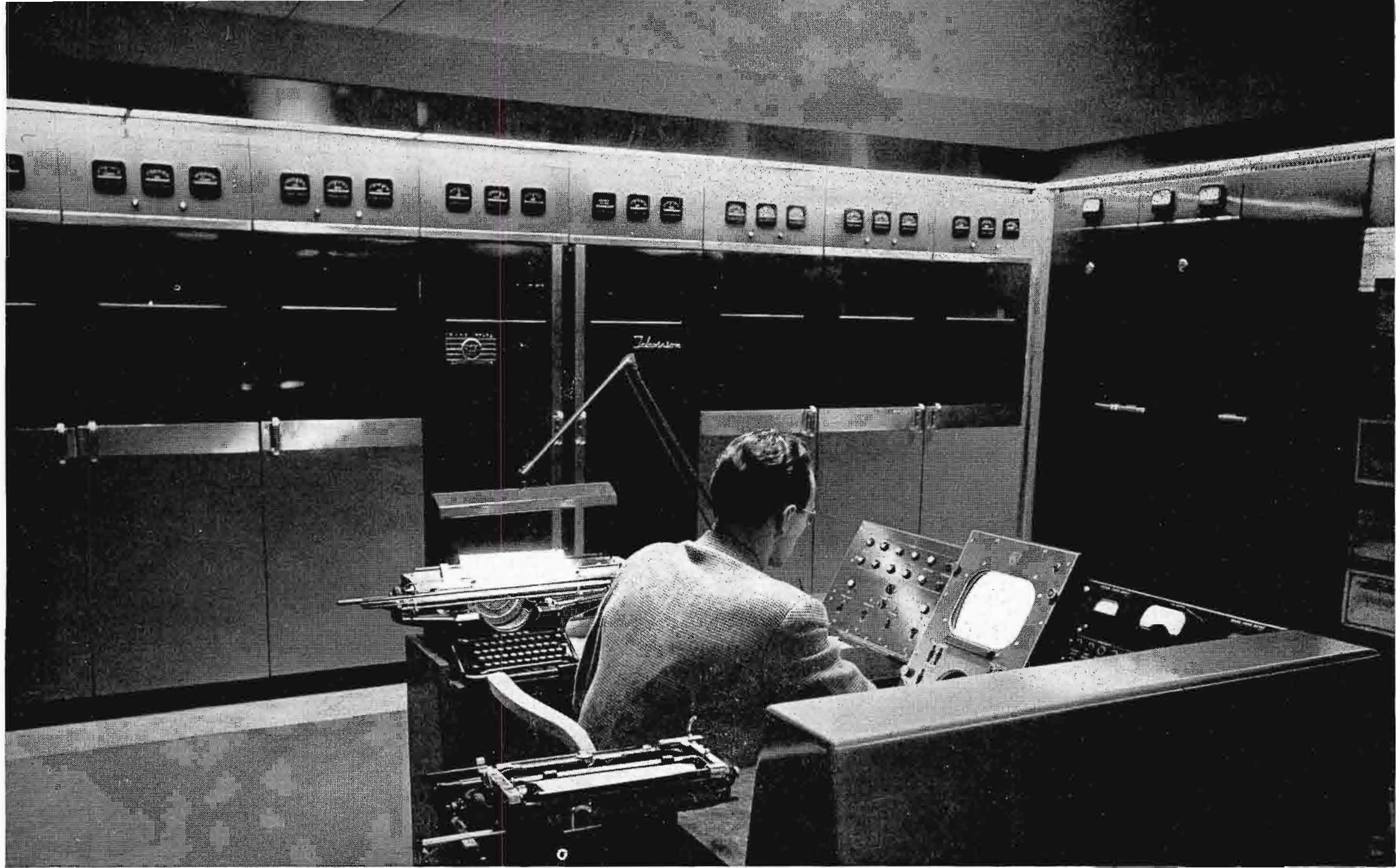
FIG. 27. WCAU-TV's Transmitter (RCA Type TT-5A) is shown here (left background). Monitoring racks are at the right, control console in the foreground. This photograph is taken from a position just in front of the FM transmitter (see floor plan, Fig. 25).
