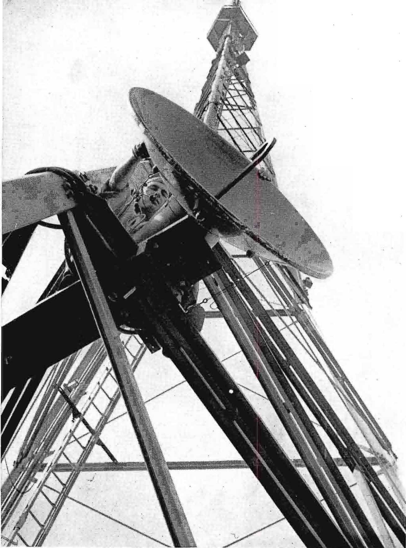
FIG. 31. WCAU-TV's exceptionally high tower is an ideal location for the RCA TRR-1A relay receiver used to pick up video signals from the mobile unit. The parabola shown above is mounted so that it can be oriented through a wide angle. Other positions provide for pickup from all directions.
