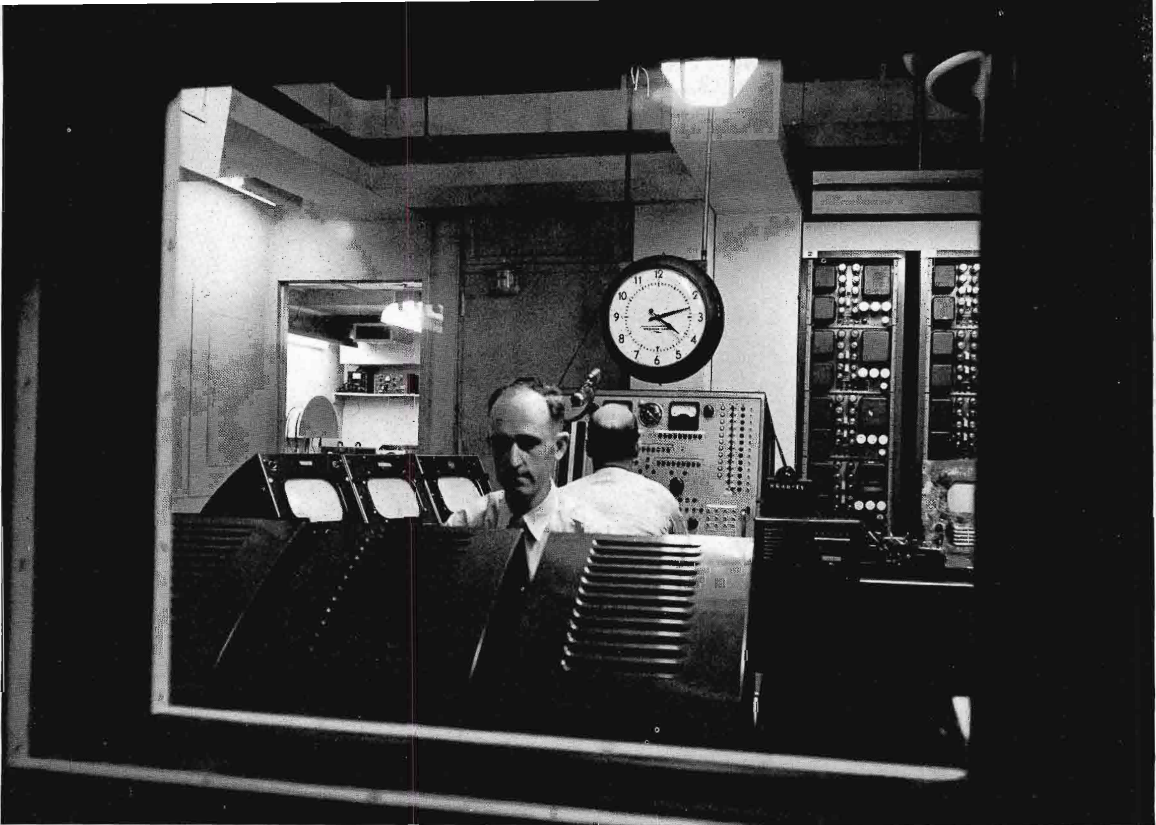
FIG. 12. The WCAU-TV Master Control Room, as seen through the window of the projection room.
