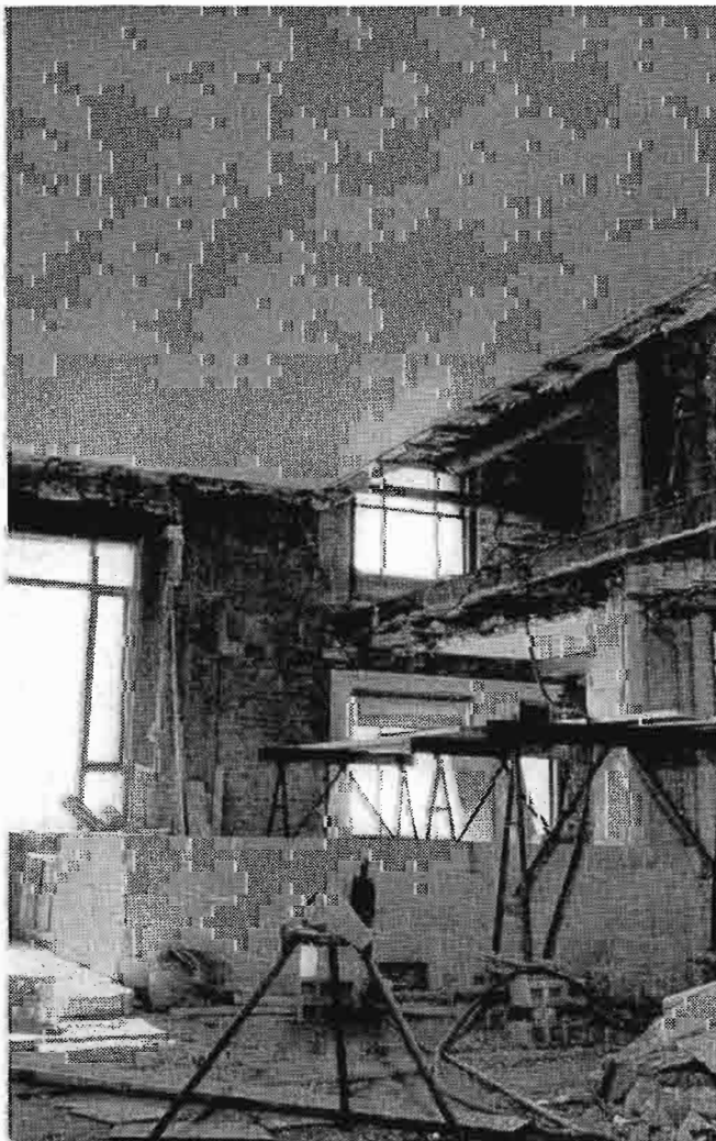
FIG. 6 (below). This is the control room corner of the penthouse studio during construction. Drop-ceiling type construction was employed in this two-story high studio.
